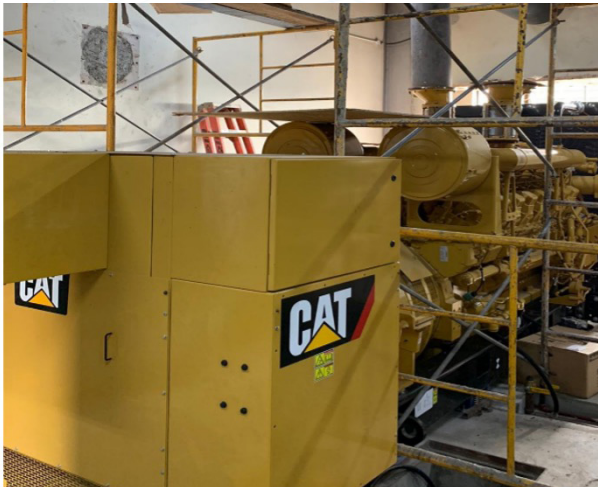
New 2MVA Caterpillar Engine Installed
