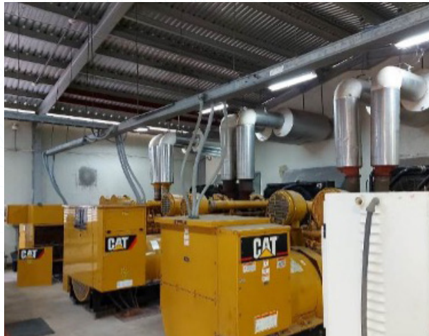
Three Generators synchronised at end of project
